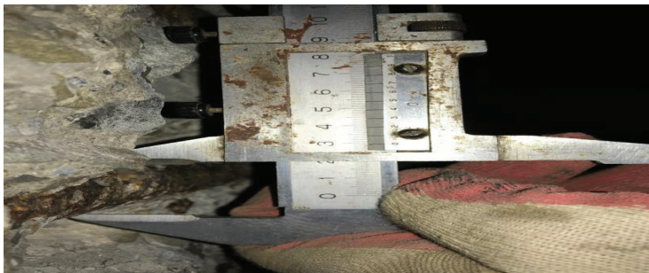
Pic. 3. Hiding the reinforcement of the rib of the floor slab above the basement
